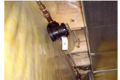
Hose Bibb Sub-metering
